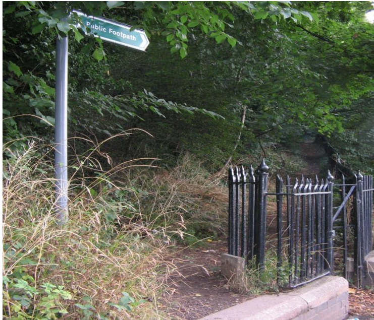
Figure 4: (before) mud washed down hill during heavy rain and collects around the gate making it virtually impossible to open. Users then had to climb up the stone wall on the left hand side
